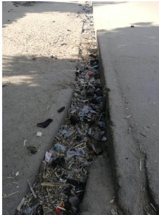
Figure 3: Drainage filled with refuse and sand
