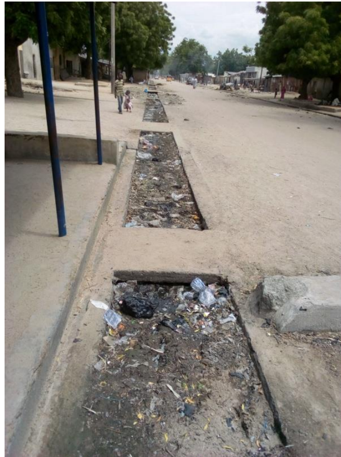
Figure 1: Open surface Drainage and Narrowed
