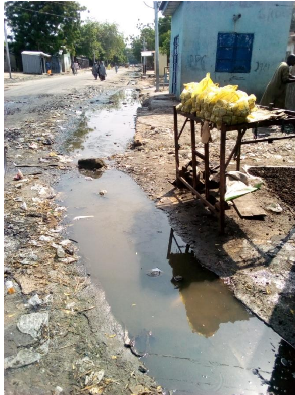
Figure 2: Drainage overflowed with sewage
