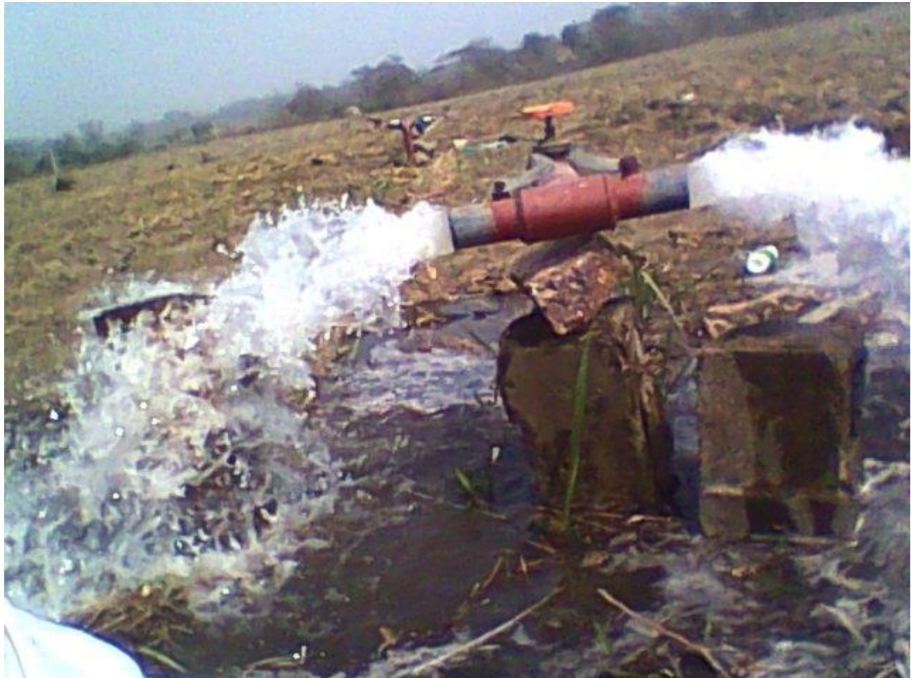
Central pump system, before hoses were inserted, at an irrigation scheme in the LNRBDA
